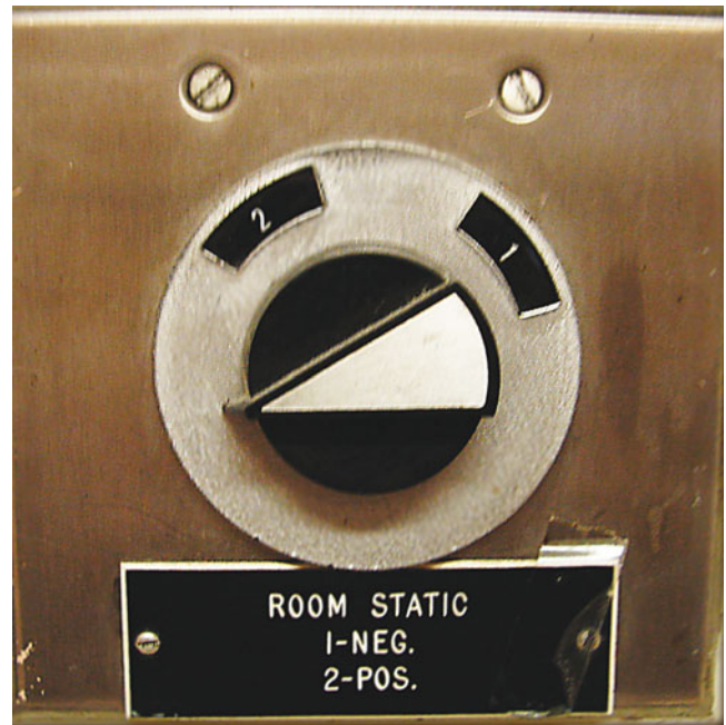
Figure 1-12. Room pressure regulator, which raises or lowers ICU room atmospheric pressure relative to the pressure outside of the room—used to partition the air in the room from the rest of the unit.
