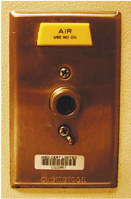
Figure 1-7. Wall air source, which is specifically color-coded yellow (in the United States) and specifically fitted for air (as distinct from oxygen) connectors and tubing.
