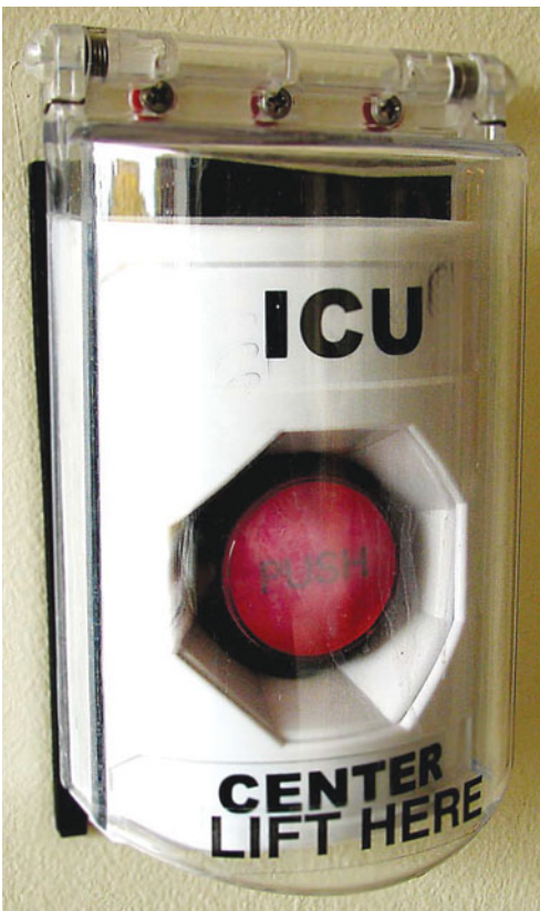
Figure 1-11. Emergency bedside “code” button which may be used to summon help in the event of an emergency.
